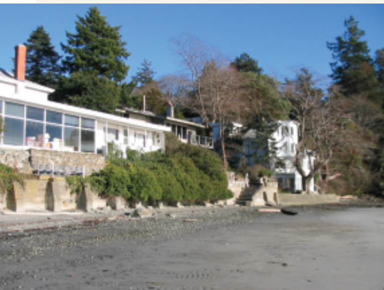
A common type of alteration of the High Water Mark to protect the property from wave erosion
